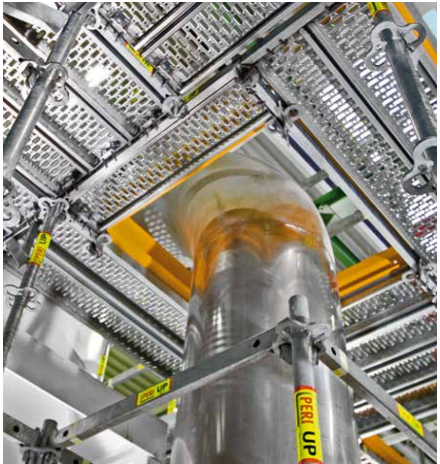
The change in direction of the decking in the 25-cm grid provides an enormous adaptability – and without any tube couplers.
